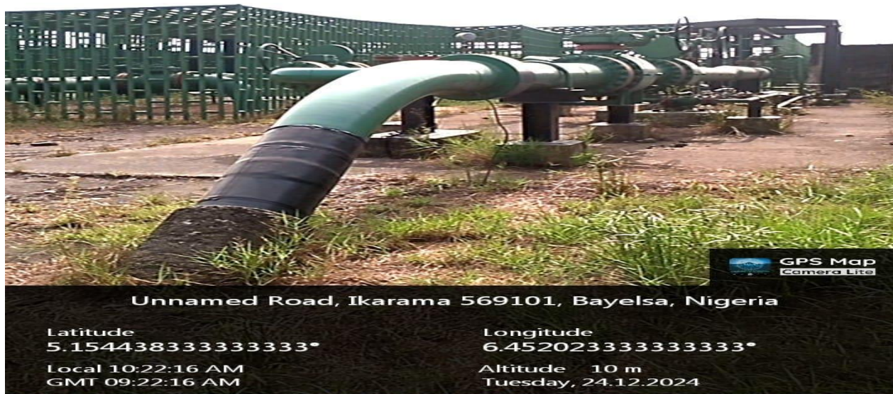
Figure 2.7: Okordia Manifold, Major Source of Illegal Bunkering in Taylor Creek Source: Author's Field Survey
