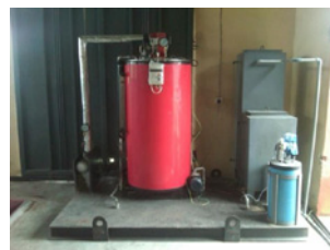
Figure 6: Steam boiler unit which produces steam for feed production.
